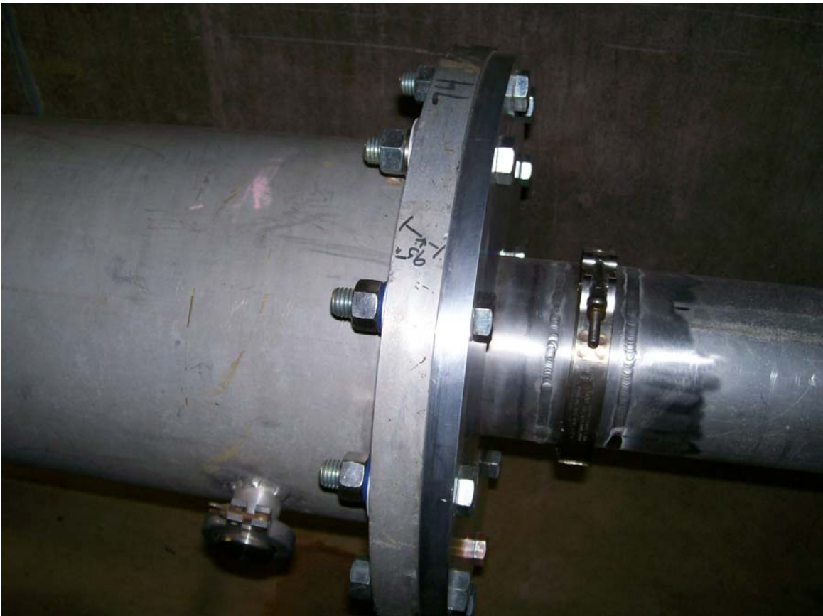
MT5CV2 UPSTREAM FLANGE
