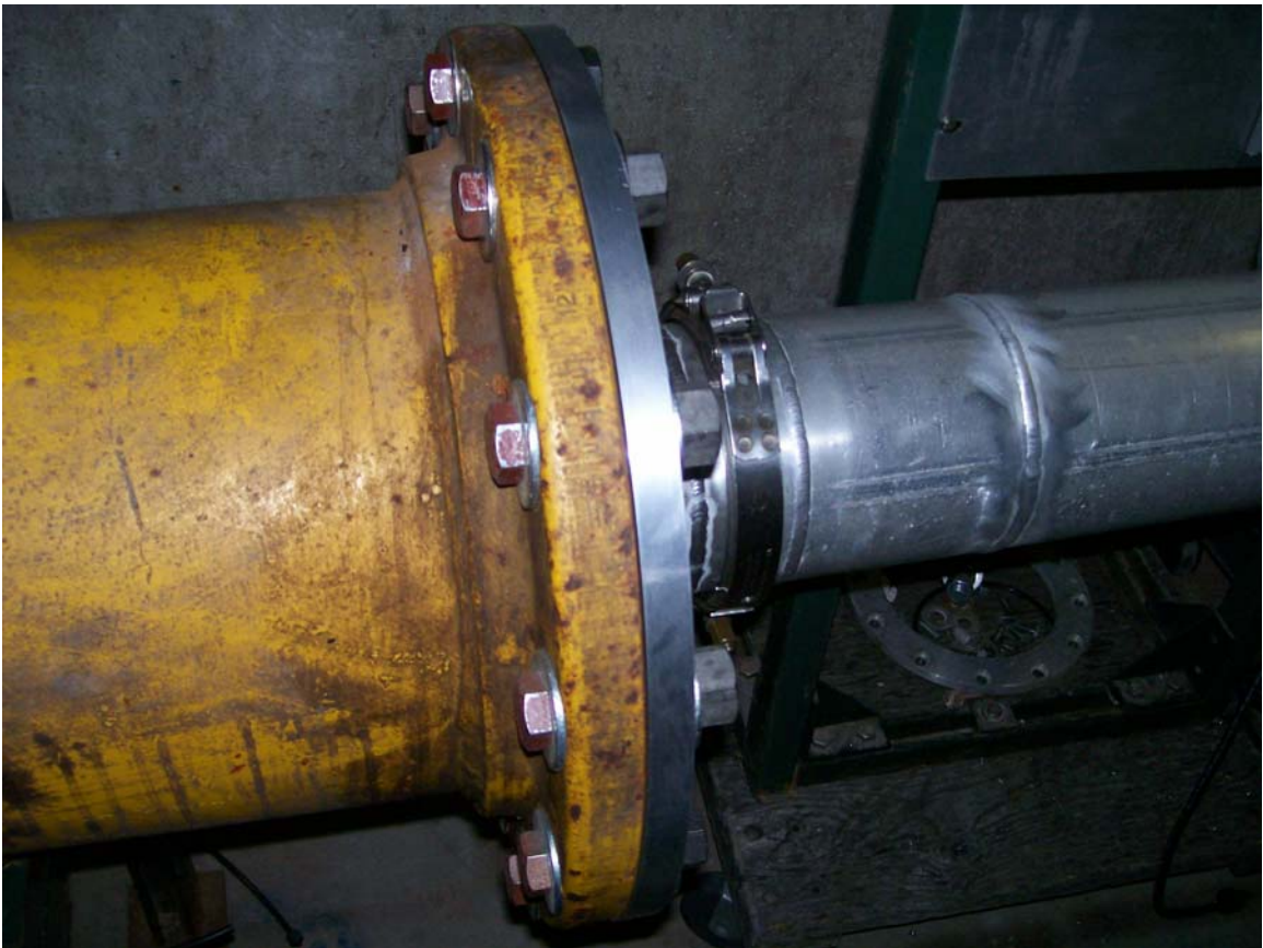
MT5CV1 UPSTREAM END
