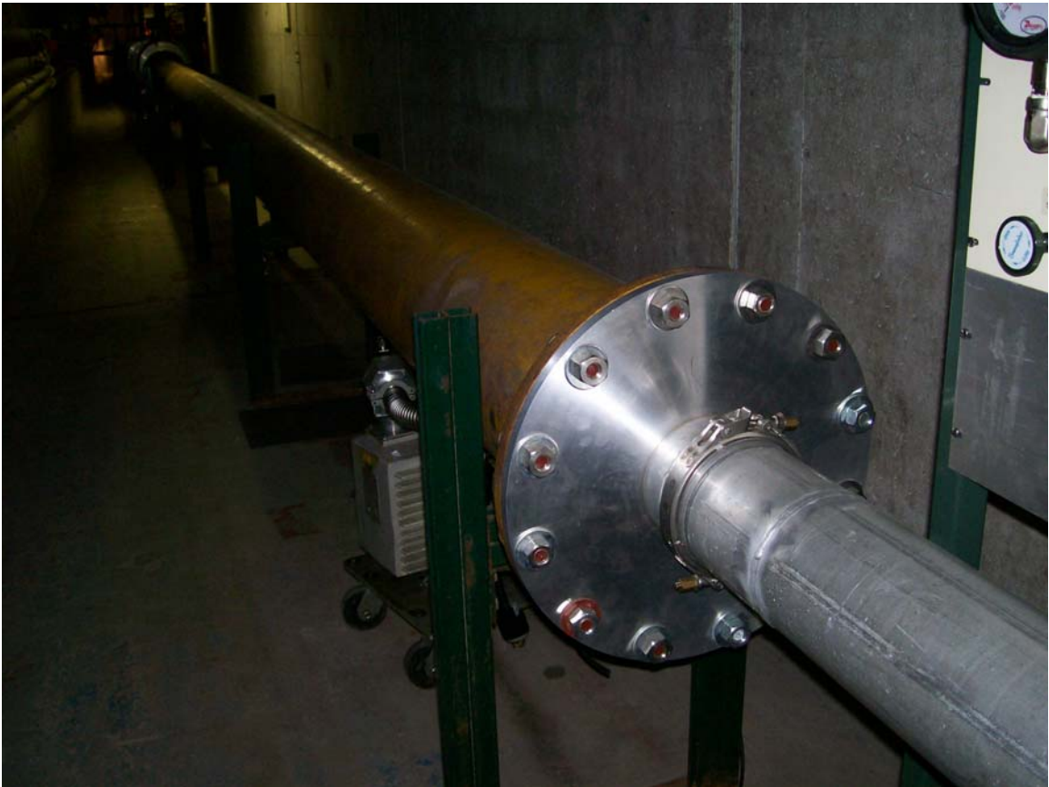
MT5CV1 UPSTREAM END
